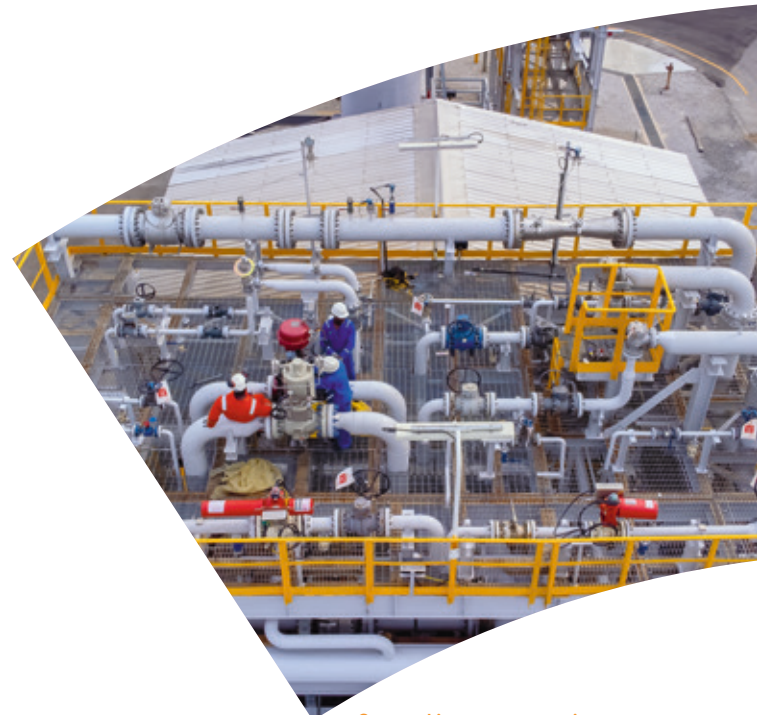
Savannah's new compression system at the Uquo CPF, Nigeria
