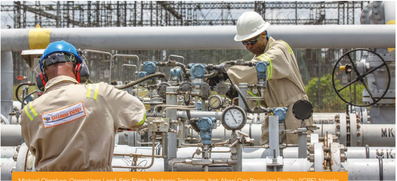
Michael Okonkwo, Operations Lead, Eric Ekine, Mechanic Technician. Ikot Abasi Gas Receiving Facility (IGRF), Nigeria.
